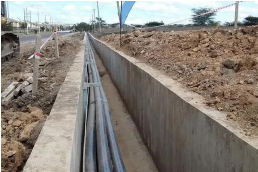
Racking in Tunnel
